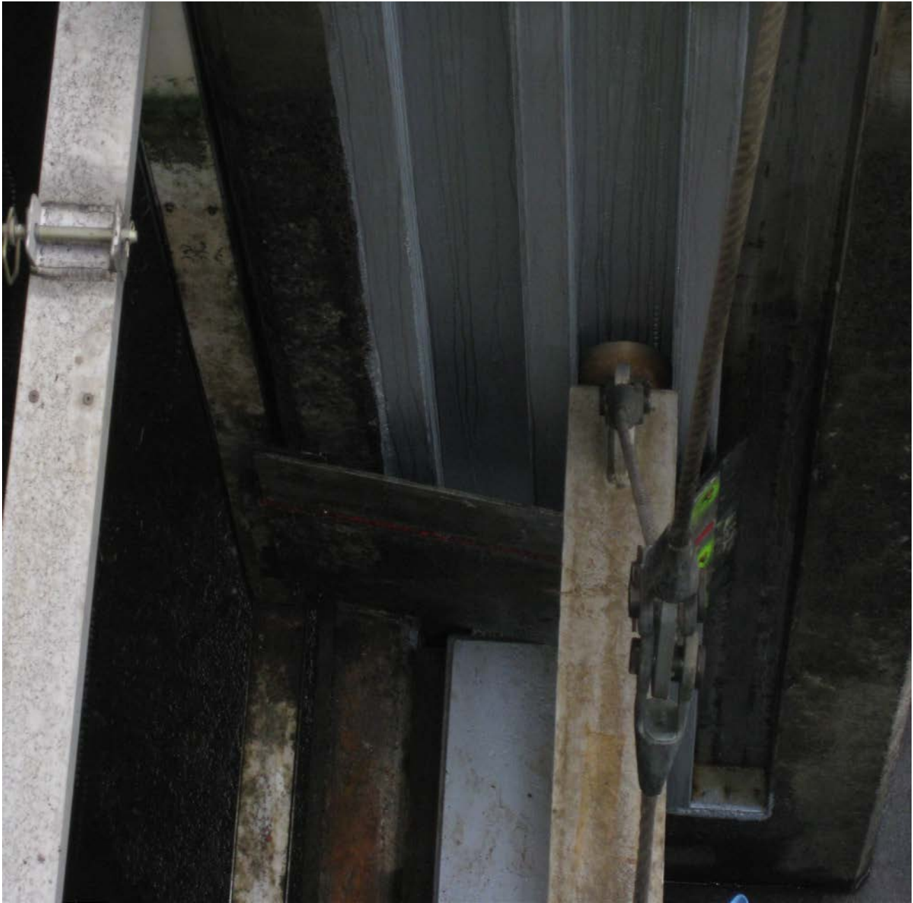
Newly installed 158 weir. Side plate touching half duplex antenna. Ogee crest cap still needs to be installed.
